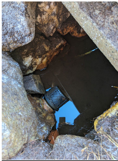
Plate 1 Tangytavil /Lagaltarve Farm PWS 02. Collection tank/chamber of collector pipes from a spring or shallow groundwater (taken February 2026).
