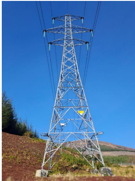
Plate 2-1: Example Steel Lattice Tower from L7 Suite
