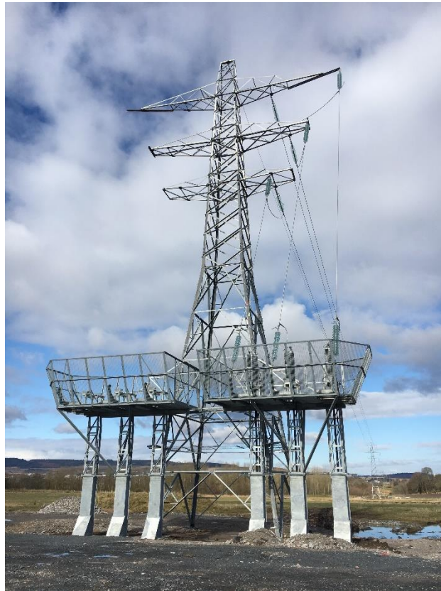
Plate 2-3: Example Terminal tower with Cable Sealing End Platform
